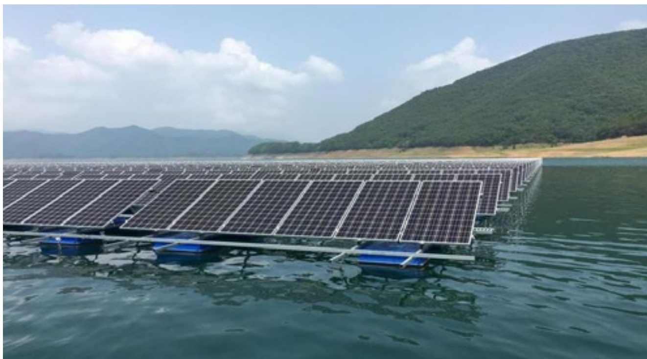
Figure 9-8 Floating solar power plant on the surface of the reservoir at Chungju Dam (Source Jecheon City Hall, January 2018)
